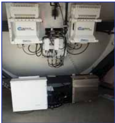
The redundant solid state and low noise amplifiers mount directly behind the antenna to the feed system. The lower support beam holds the antenna motor control cabinet and regenerative dehydrator.
