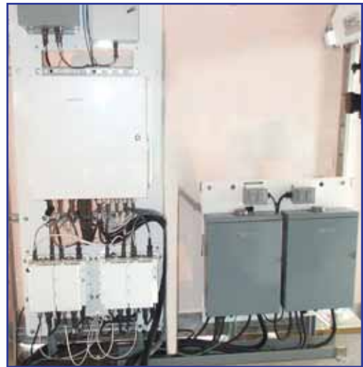
The Outdoor Equipment Assembly is co-located with the antenna in the radome. This frame includes the Outdoor Signal Enclosure, Block Up Converter, Block Down Converter, Test Loop Translator, Intercom, and Technical and Utility AC Power Panels.
